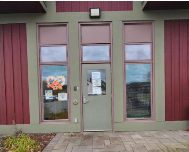
Side Entrance Exterior- Right and Left windows are included in Windows list
